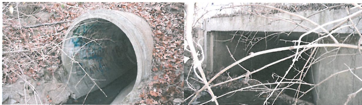
Figure 1: Photos of the Deficient Culvert (Left, Downstream end section: Right, Upstream end section)
