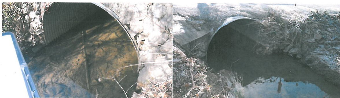
Figure2: Photos of the undersized culvert (Left, Downstream end section; Right, Upstream end section)
